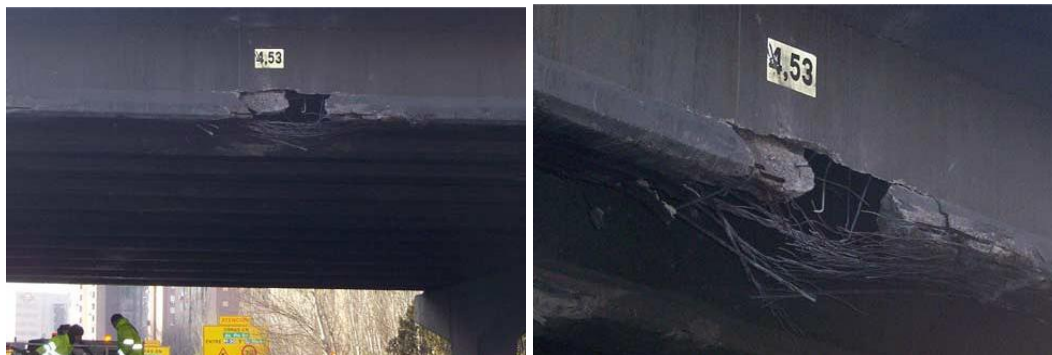
Fig. 2-5: Collision of an oversize load truck with a prestressed girder bridge in Madrid, Spain (elmundo.es, 2005).
