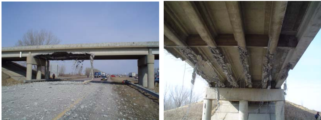
Fig. 2-6: Damage to a prestressed girder bridge caused by a truck in Iowa on 2005 (source is unknown).
