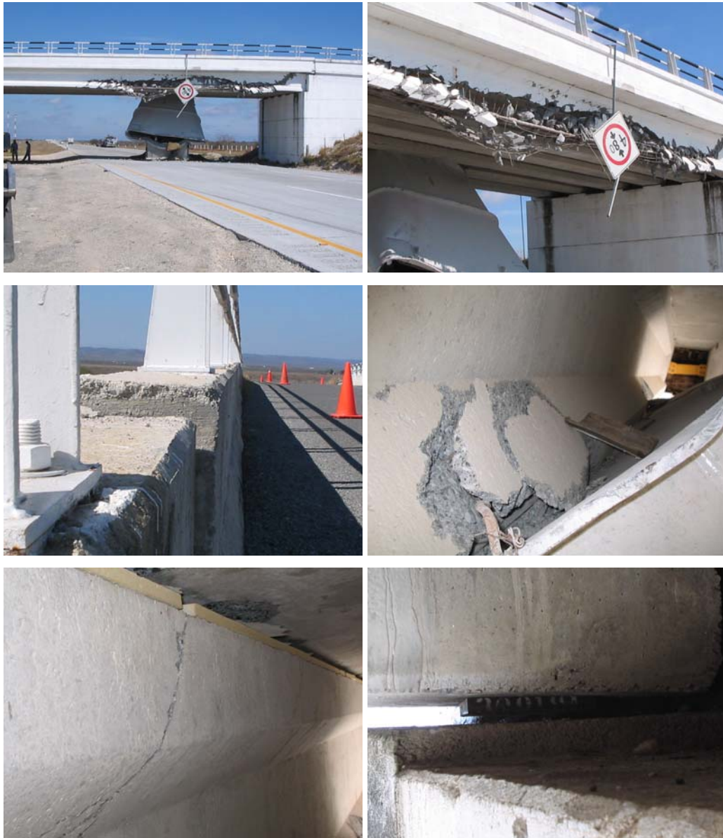
Fig. 2-7: Damage to a prestressed girder bridge caused by a truck near Monterrey, Mexico on 2005 (courtesy of Gutierrez Ingenieros).
